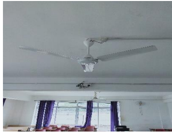
Celing & Wall fans (12 Nos)
